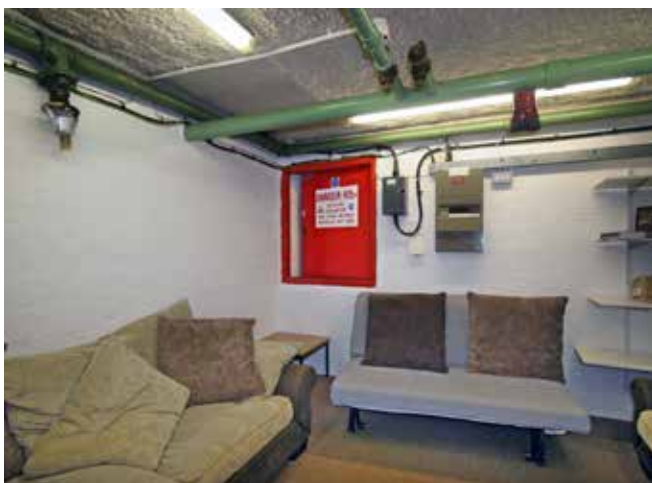
The emergency generator is located through this high level door located at the rear of the government departments room
